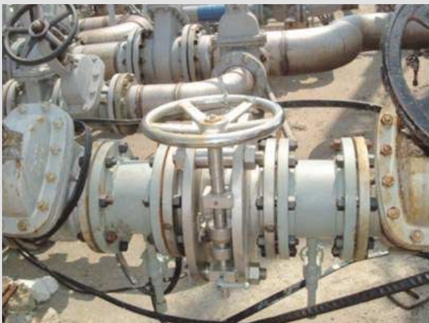
■ Naptha feed line of cracking heater for Ethylene plant
